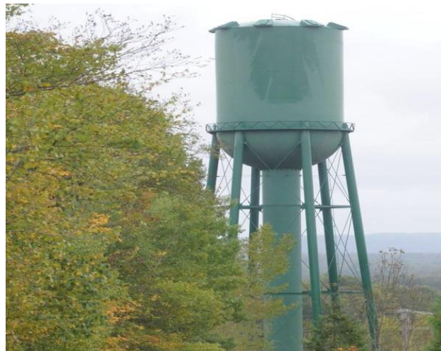
Figure: Surge Tank
